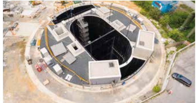
Pumping station in Gelsenkirchen
