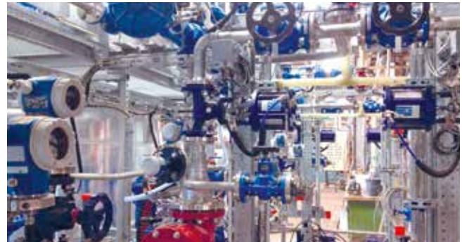
Wastewater treatment plant in Ruhleben. Flue gas purification unit
